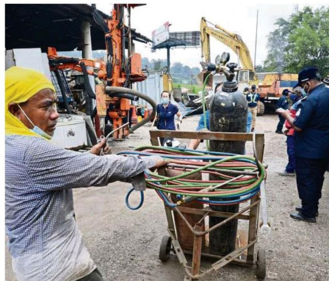
A worker removing equipment from a heavy machinery workshop as the excavator's claw came crashing down on illegal business premises.
