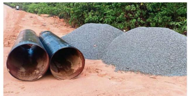
A check by StarMetro found piles of gravel and steel culverts at the site. — Filepic
